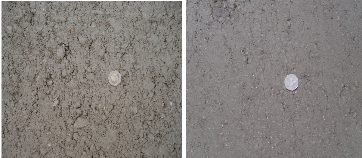
Figure 1: Typical surface finish with 20mm (left) and 10 mm (right) maximum aggregate size
